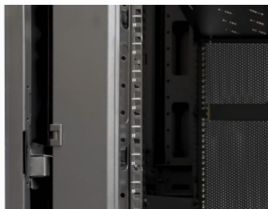
Vertical Cable Management Rails Opened
