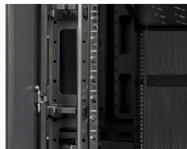
Vertical Cable Management Rails Closed
